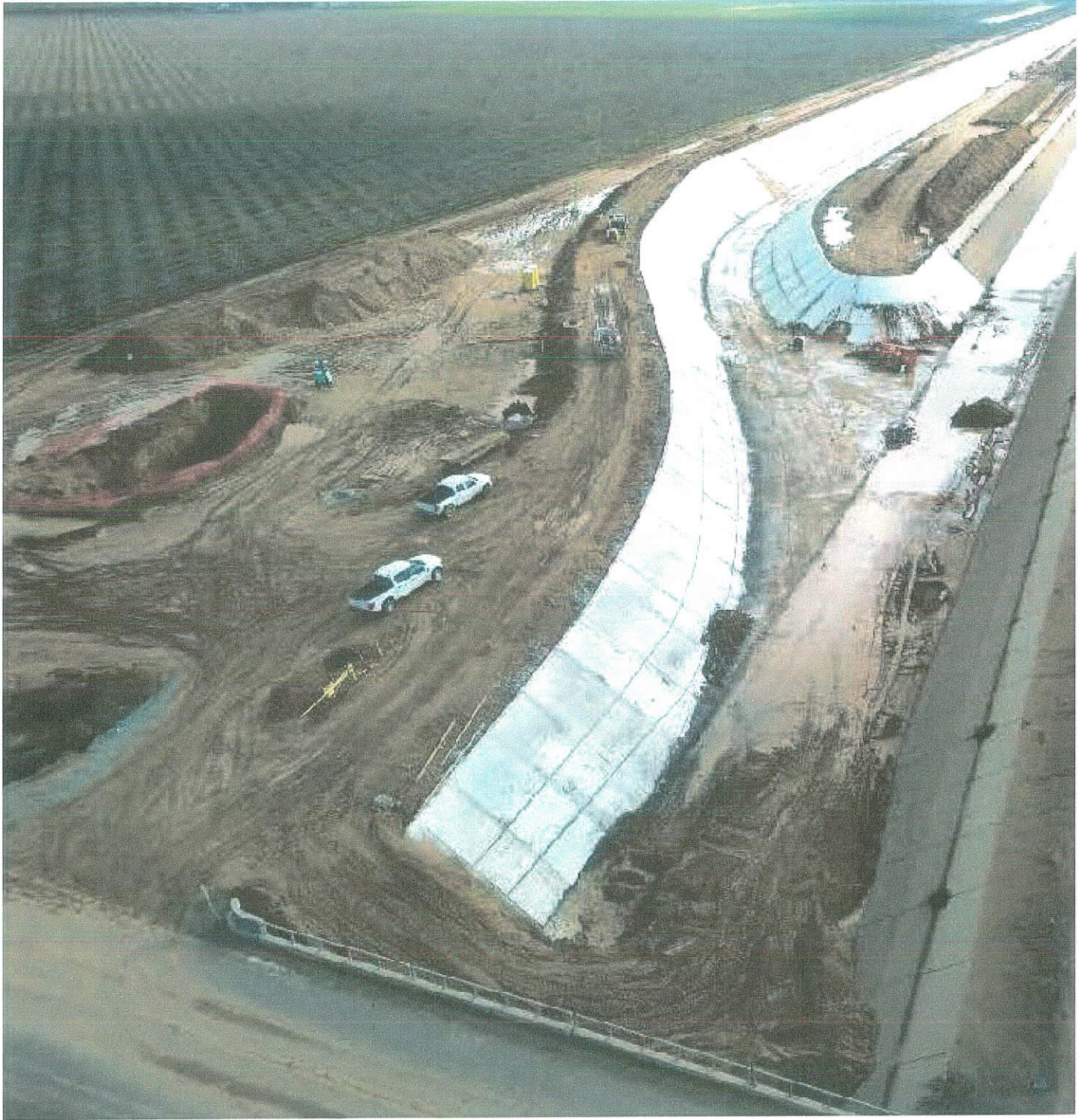
Construction on the Friant-Kern Canal shows a new canal being laid out next to the existing canal, which has sunk due to overpumping groundwater in the region. (Friant Water Authority)
